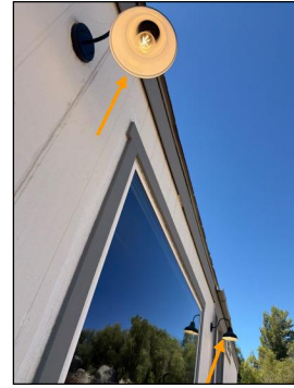
Out door lamps operational
