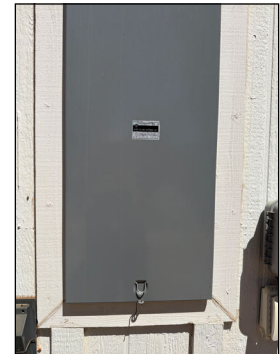
Sub Panel Exterior
