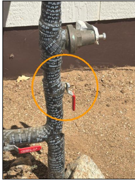
Main Water Shut Off Valve
