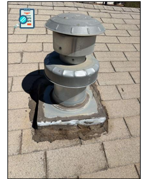
Small gaps in sealant recommend reapplying in needed areas
