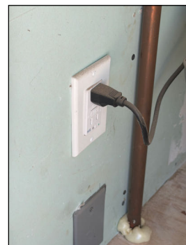
Heater Electrical Disconnect
