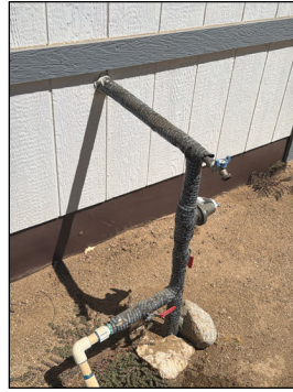
Piping concealed with PVC tape
