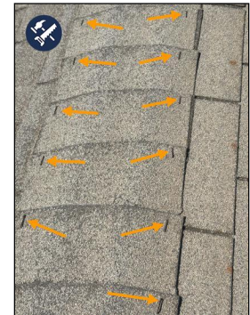
Staples in one or more shingles not sealed
