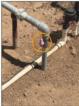
Main Gas Shut off Valve
