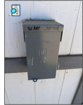
Hot Tub disconnect (recommend asking owner about the panel and its receptacle location for reference)
