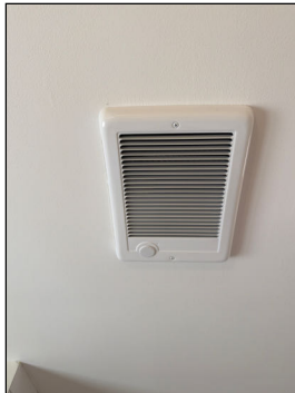
Heater in each bathroom
