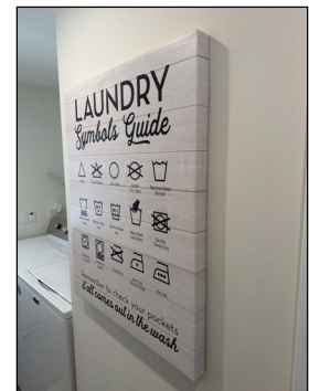
#2 Sub Panel Behind this frame
