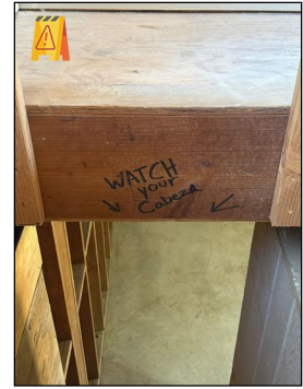
Low Header noted
