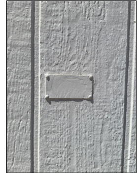
HUD Label (not visible painted over)
