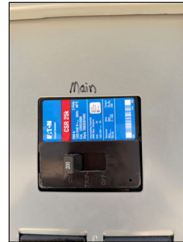
#2 Sub Panel Main Breaker 200amp
