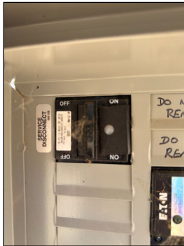
Main Panel Breaker 200amp
