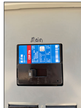
#2 Interruptor principal del subpanel 200amp
