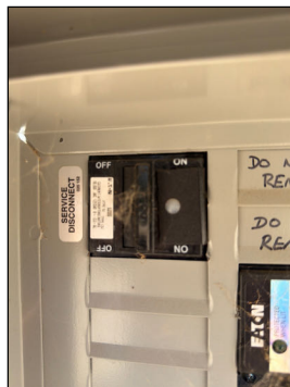
Interruptor principal del panel 200amp
